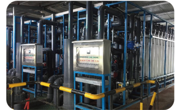
印染废水零排放项目 Printing and dyeing wastewater zero discharge project
