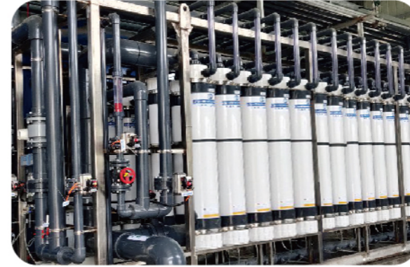
钢厂水处理工程 Steel mill water treatment project
