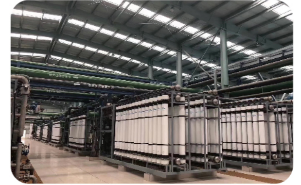
钢厂水处理工程 Steel mill water treatment project
